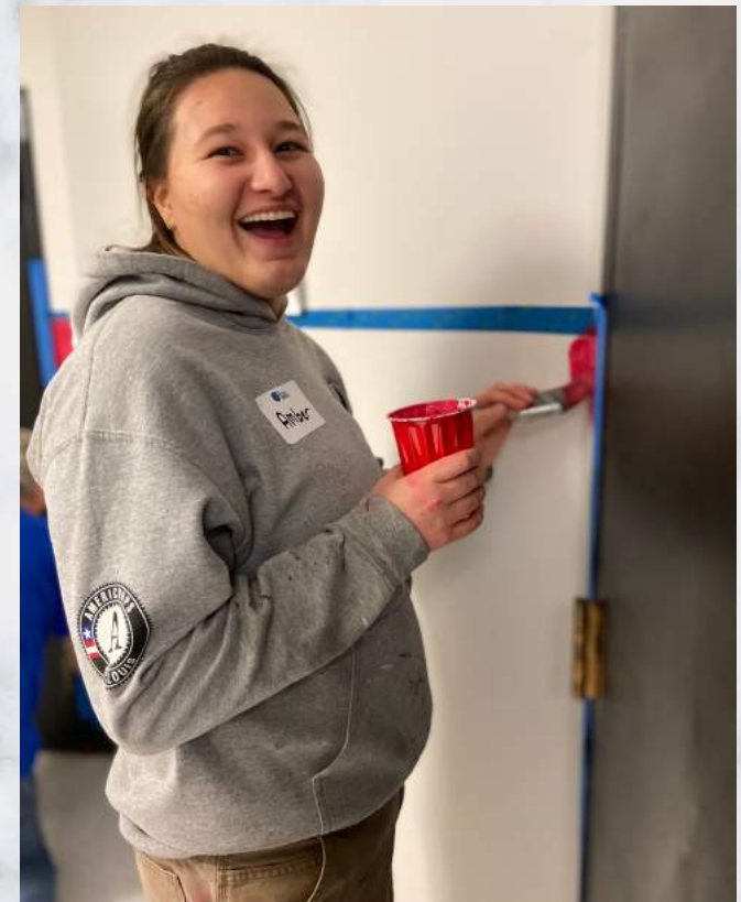
Amber Andrews paints a wall at Twillman Elementary School for Martin Luther King Jr. National Day of Service project with The Mission Continues.
